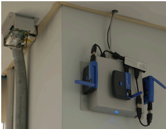
Fig. 2. Bottom right: WiSEMesh node deployment in the office building. Top left: Sensor network node.
